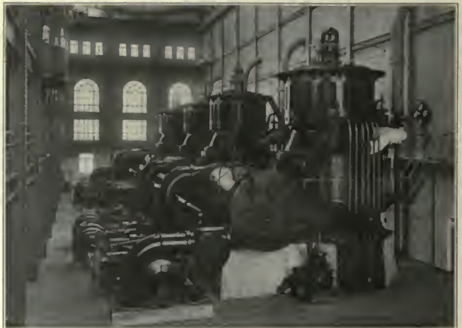
FIG. 489. POWER STATIONS. Interior View, Port Morris Power Station of the New York Central & Hudson River Railroad. Capacity, 20,000 kw.
